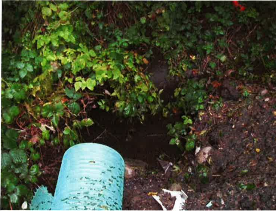
Photo 7: Brydon Creek. Culverts on downstream side of 55A Avenue. Location of reduced fish passage
