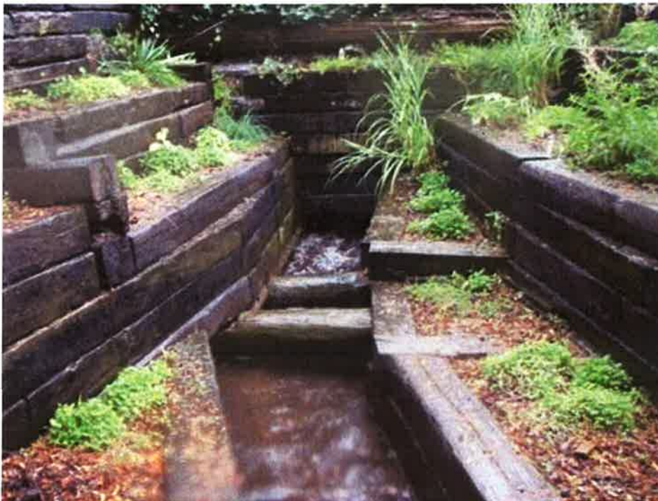
Photo 17: Tributary to Nicomekl River; upstream of convergence with Langley Creek. Creosote barrier structure at 4850 206 Street
